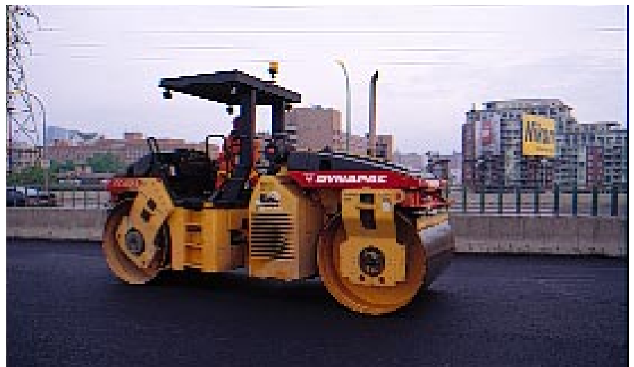
A Dynapac CC 422 tandem-drum unit making a breakdown pass on the Gardiner Expressway job.
