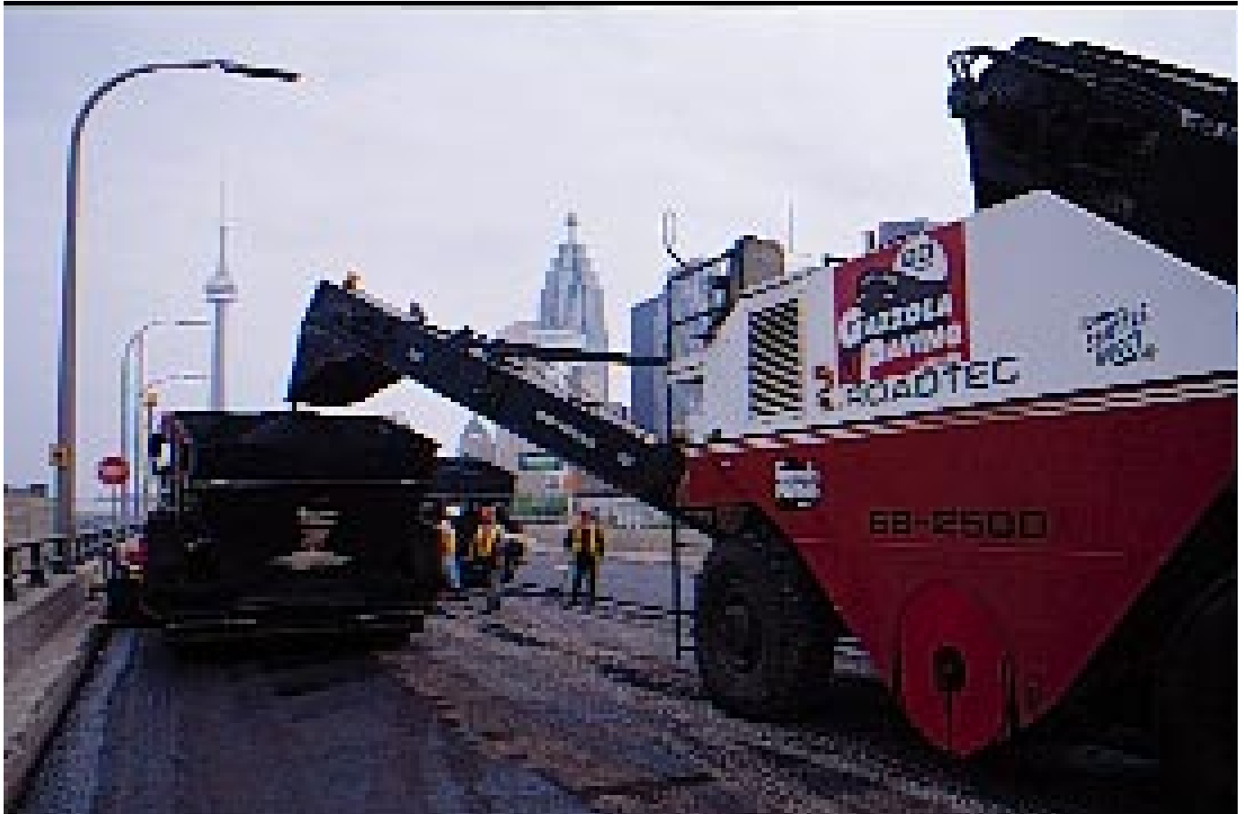
Gazzola's paving crew achieved a laydown rate of an average laydown rate of 280 tonnes-h on this high profile job with a Roadtec SB 2500 Shuttle Buggy and two Caterpillar AP 1055B pavers.
